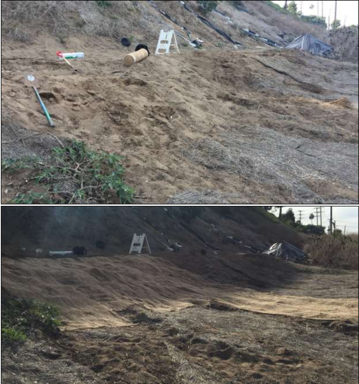
Figure 23. Photographs taken of the impacted area of the hillside with disturbed soils and tracks before emergency measures were taken (top) and after erosion control mats were placed (bottom) (26 November 2019).
