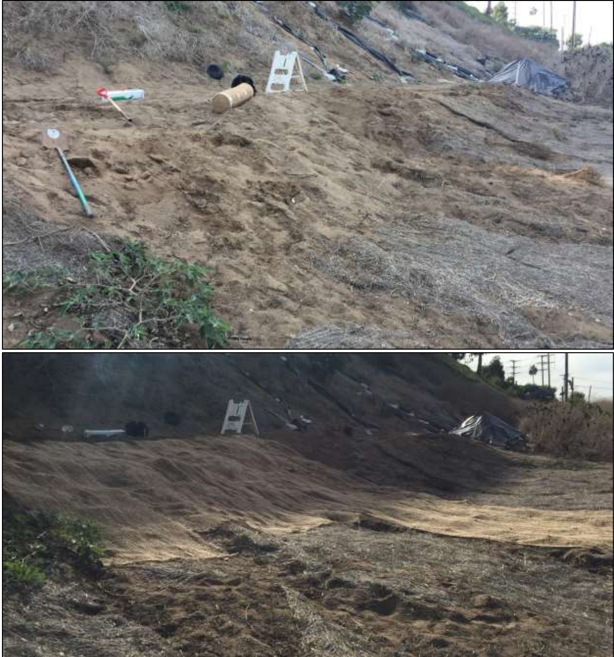
Figure 23. Photographs taken of the impacted area of the hillside with disturbed soils and tracks before emergency measures were taken (top) and after erosion control mats were placed (bottom) (26 November 2019).
