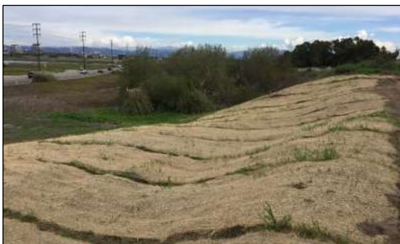
Figure 2. Hillside in restoration area following weeding, seeding with native coastal upland species, and installation of erosion control mats on 21 February 2019.
