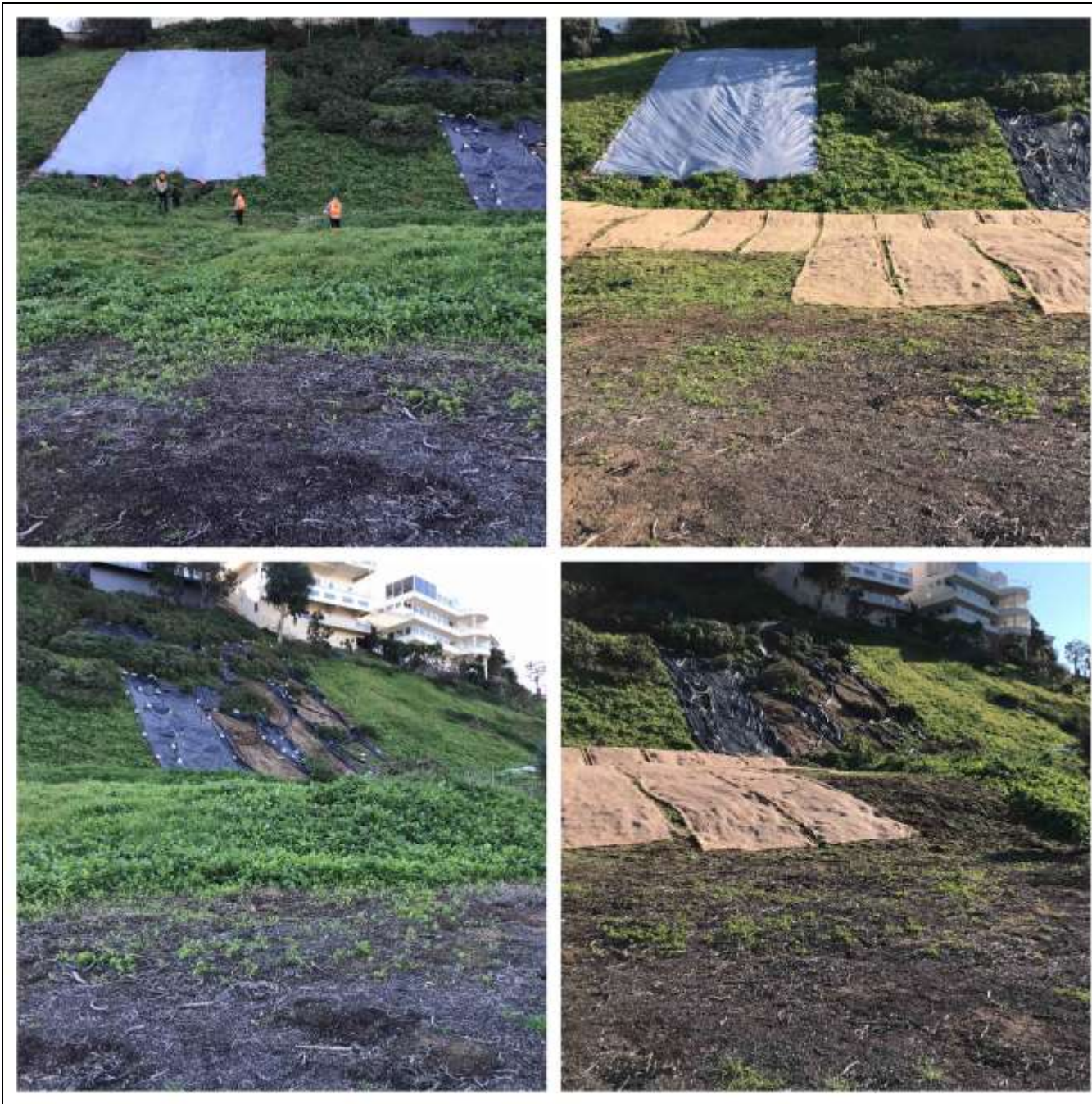
Figure 45. Hillside before and immediately post weeding, seeding, and erosion control mat installation on 8 February 2019.
