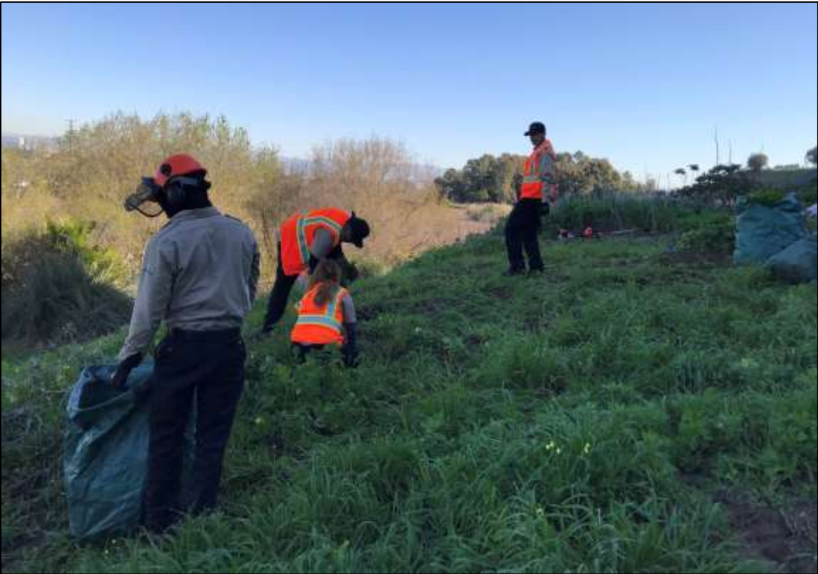
Figure 8. Los Angeles Conservation Corps and TBF conducting site preparation, seeding, and erosion control installation on 8 February 2019.
