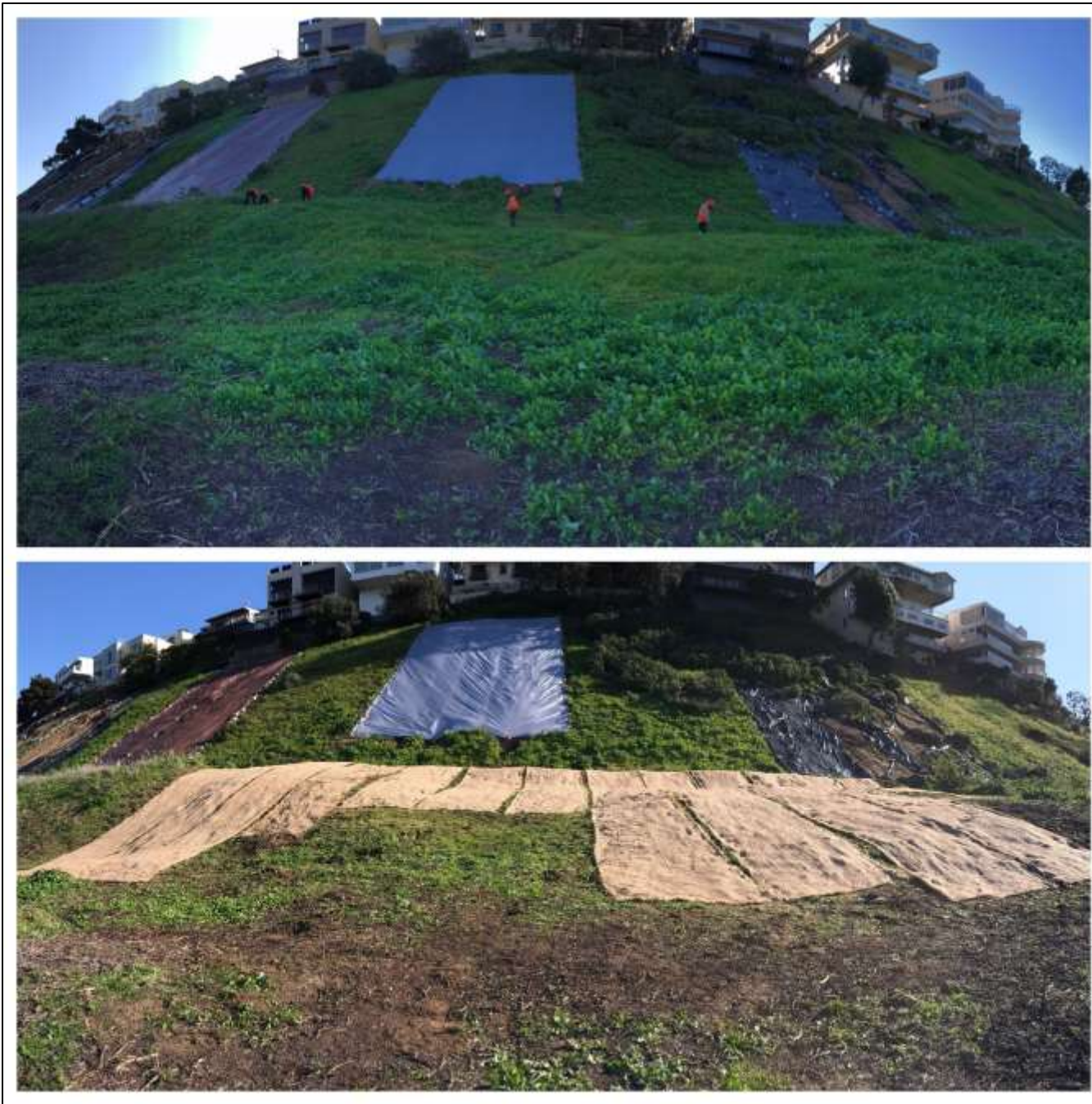
Figure 46. Hillside before and immediately post weeding, seeding, and erosion control mat installation on 8 February 2019.
