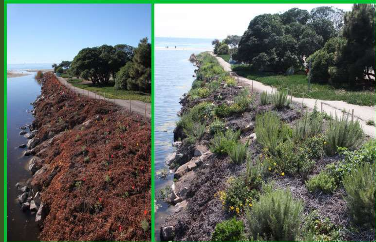
Project site (looking south) after removal of plastic sheeting and initial installation of native plants.
