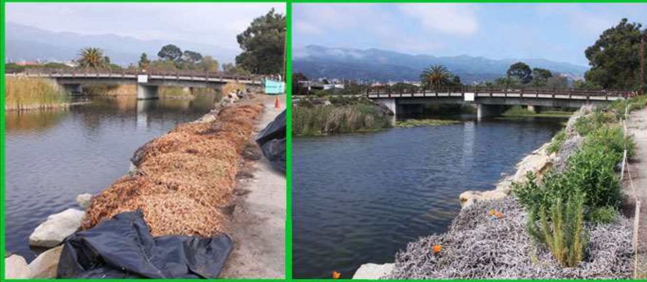
Project site (looking north) after removal of plastic sheeting and initial installation of native plants.
